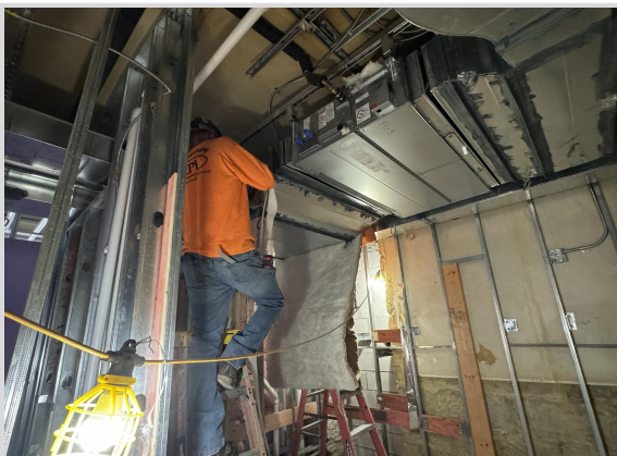
Ground Floor Duct Insulation 11/22/24
