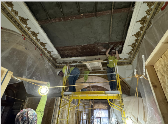
1st Floor Parge Coating 11/27/24
