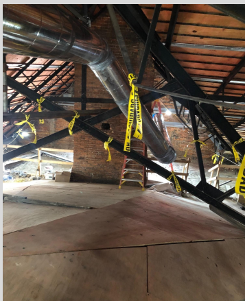
HVAC Duct Installed In The Attic 8/9/24
